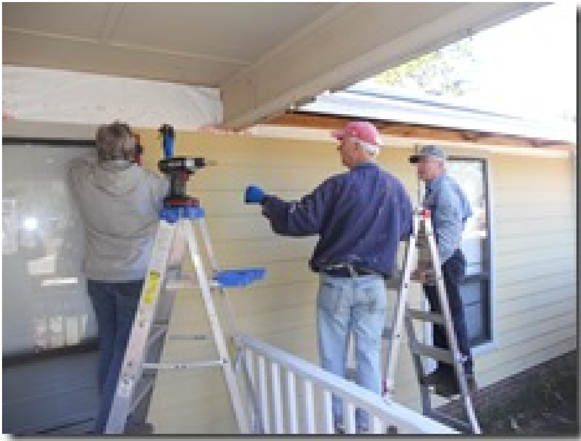
Gerri Tulley, Dick Grier, and Dale Sticka continue to replace hardy board siding on the house.
