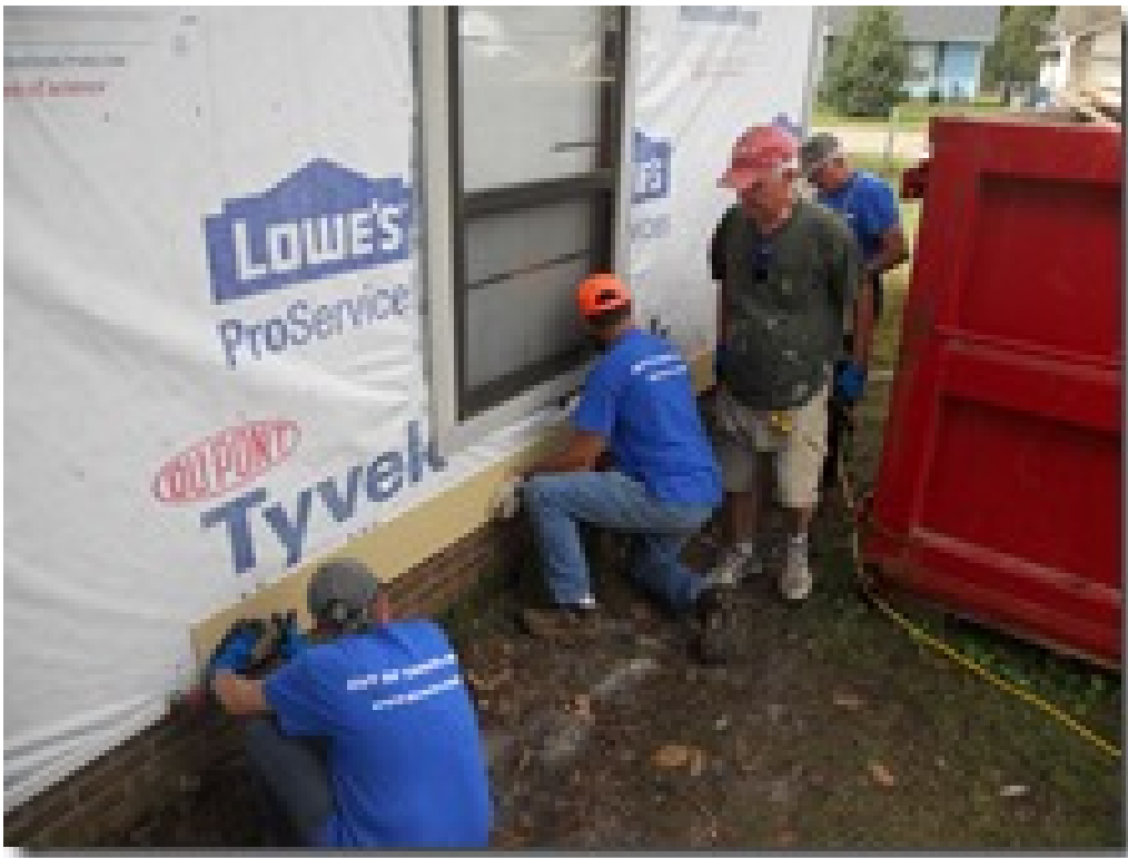
Gerri, Phil Trick, and Dale Sticka begin replacement of the new hardy board siding on the house.
